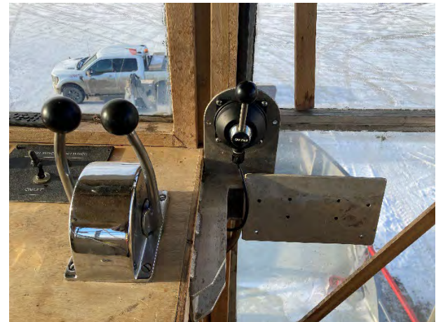
ITEM #37 Broken Jog Stick Replaced
