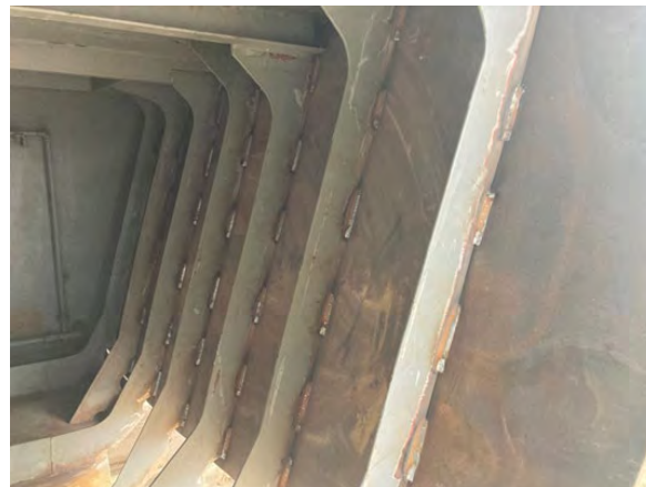
ITEM #3 Internal Port Renewed Stitching on Ribs
