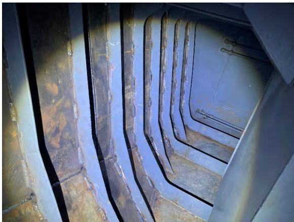
ITEM #3 Internal Starboard Renewed Stitching on Ribs
