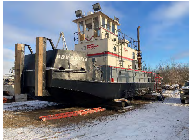
ITEM #41 Push Knees Replaced with new lumber
