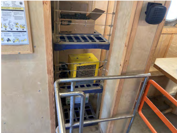
ITEM #40 Heater Installed in Galley
