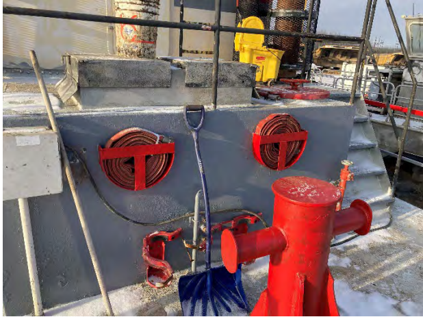
ITEM #38 Fire Hoses old and worn out replaced
